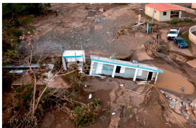
Damage in Puerto Rico from the latest in a series of relentless natural disasters.
